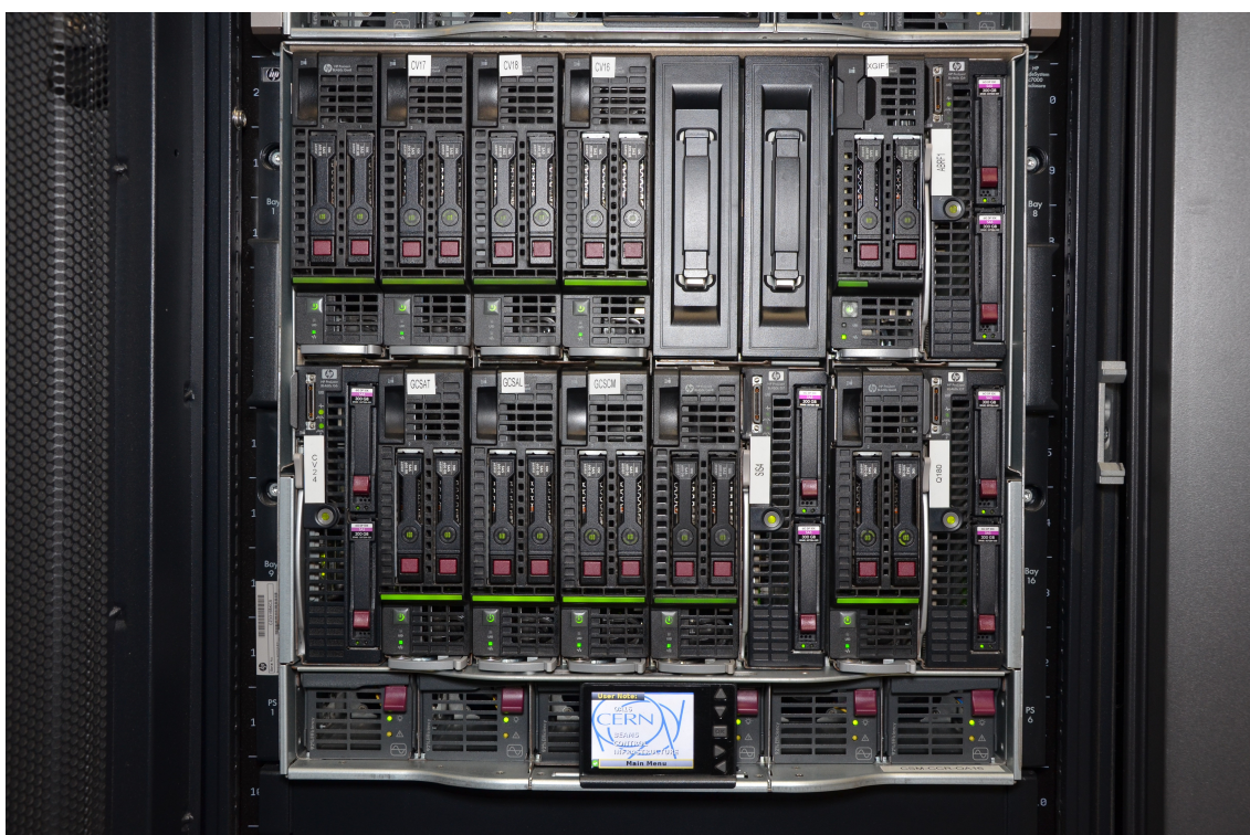
Figure 1.3: 19-inch enclosure with 14 servers running the controls business logic
